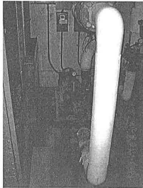
Photo 5 – Heating Pump for Addition
