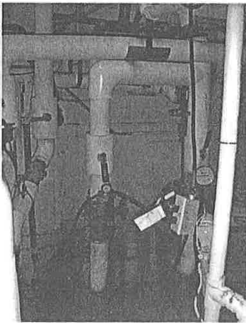
Photo 4 – Existing Heating Pumps
